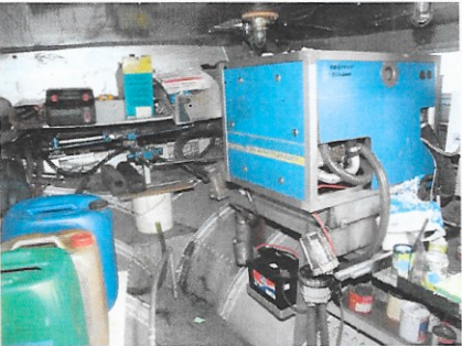
Generatorset in the workshop
